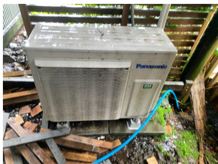
Exterior Heating system/condenser Heat pump, Panasonic CU-RZ7IVKR View High Resolution Image Here
