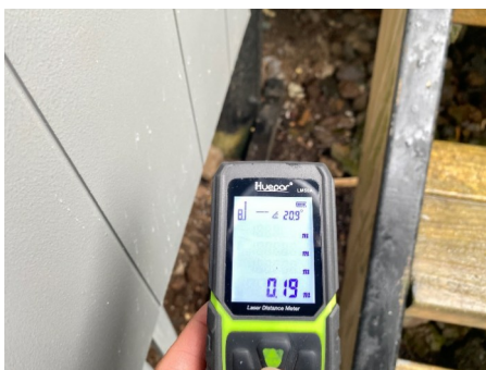
Subfloor access Access too narrow and blocked. View High Resolution Image Here
