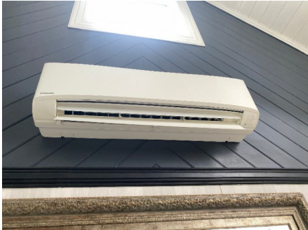
Heater Heat pump, Panasonic CU-RZ7IVKR Current heater in good working condition. View High Resolution Image Here
