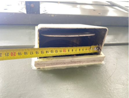
Bathroom 1 extraction system ducting Ducting measurement is 150mm. View High Resolution Image Here
