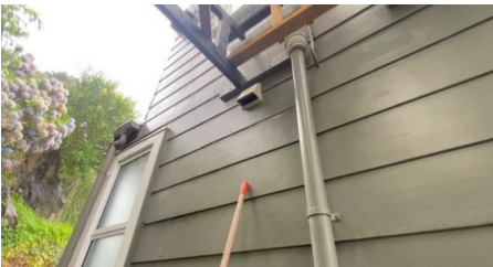
Bathroom 1 extraction system external vent Confirmed by smoke test. View High Resolution Image Here
