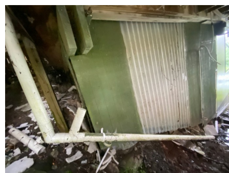
Rear of property - downpipe Downpipe not connected to an appropriate outfall. View High Resolution Image Here
