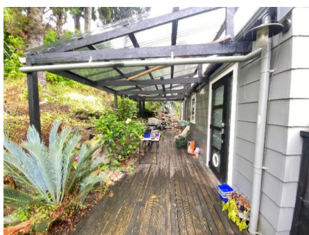
Rear of property - downpipe Downpipe not connected to an appropriate outfall. View High Resolution Image Here
