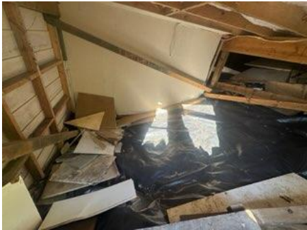
Moisture Barrier remediation View High Resolution Image Here 02/02/2026
