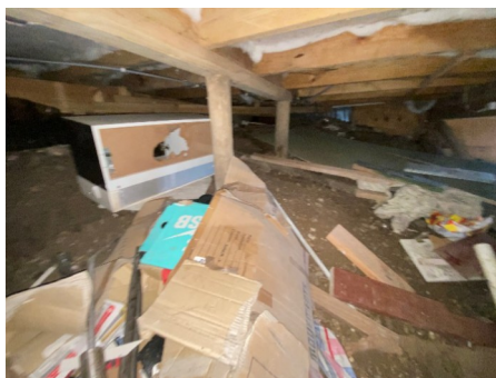
Sub floor internal context No moisture barrier has been installed in the sub floor. View High Resolution Image Here
