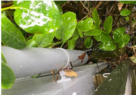
Front of property - downpipe Downpipe not connected to an appropriate outfall. View High Resolution Image Here
