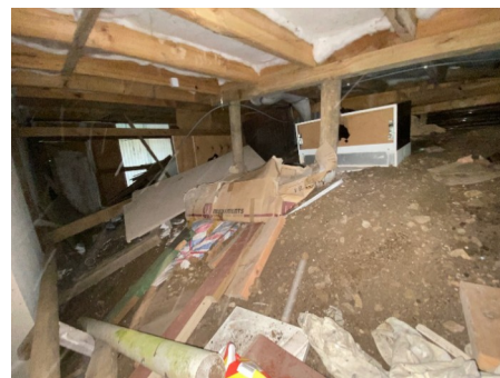
Sub floor internal context No moisture barrier has been installed in the sub floor. View High Resolution Image Here
