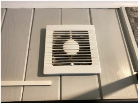
Bathroom 1 extraction system The extraction system is in good working condition. View High Resolution Image Here
