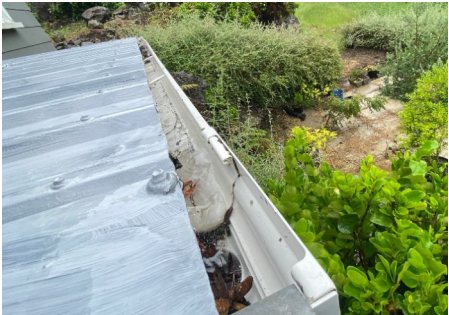
Front of property - spouting Spouting is blocked by plants or debris preventing effective drainage. View High Resolution Image Here
