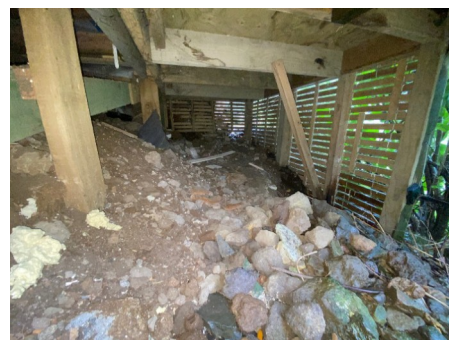
Sub floor internal context No moisture barrier required, Access too narrow and blocked. View High Resolution Image Here
