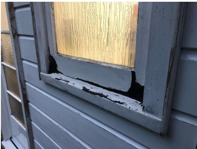
The window casement should be filled and paint coat sealed to prevent moisture ingress.
