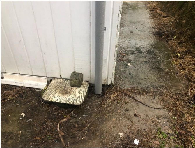
Example. The downpipes are currently discharging directly at the base of the building envelope.
