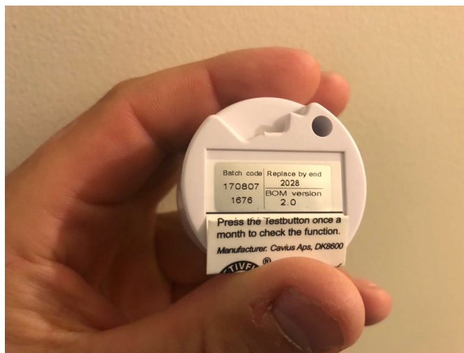
Qualified smoke detector noted and tested. Expiry 2028
