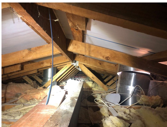
The existing ceiling insulation has significantly slumped over time below the minimum requirements to meet the insulation standard. A top up layer of insulation should be applied however It is this inspectors opinion that the ceiling cavity height is well below the minimum standard for access to install ceiling insulation. In this instance exemptions have been applied.
