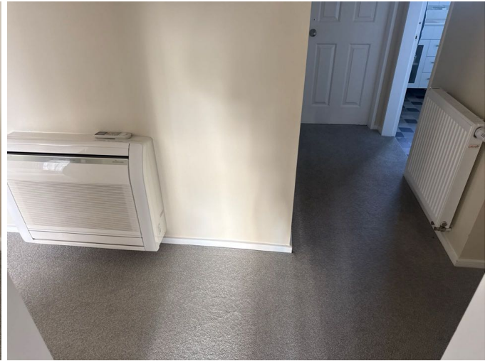
Heatpump and radiator to the hallway
