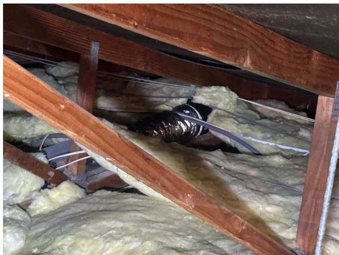
Extraction units vent to the exterior
