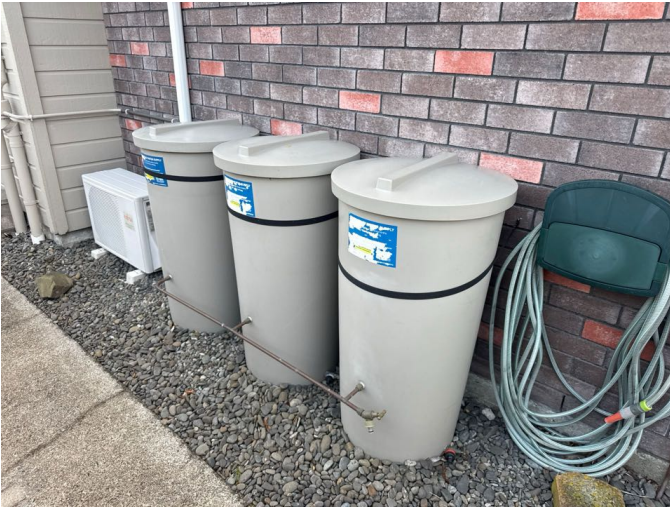
Water storage tank installed on the southwest side
