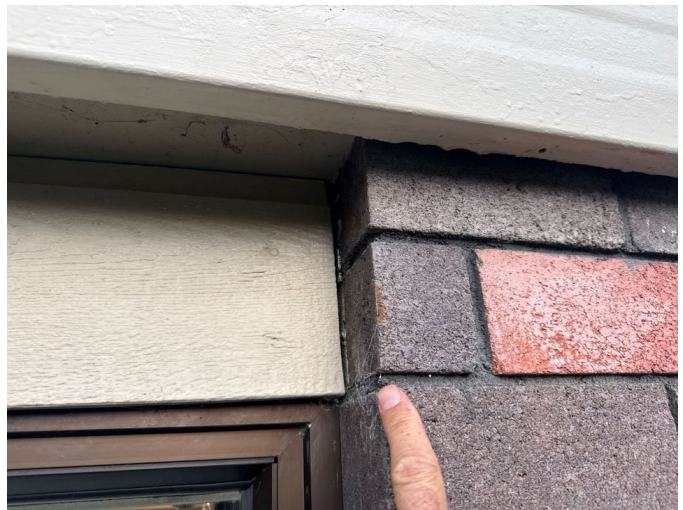
Gaps like this above the windows between the weatherboard and the brick should be sealed.
