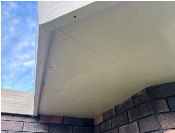
There is visible evidence of previous overflows into the soffit from the internal gutters. Replacing this system is the best long term improvement option (recommended by T.H.I.S).
