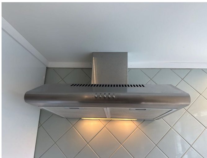
The range hood extraction unit is functioning
