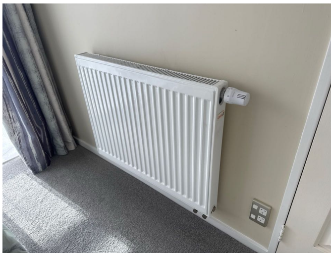
Radiator heating to the bedrooms
