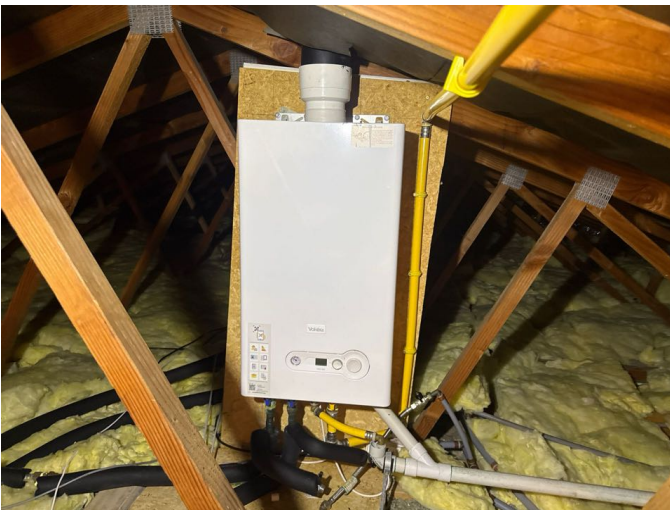
The boiler for the radiator heating system is located in the ceiling cavity.
