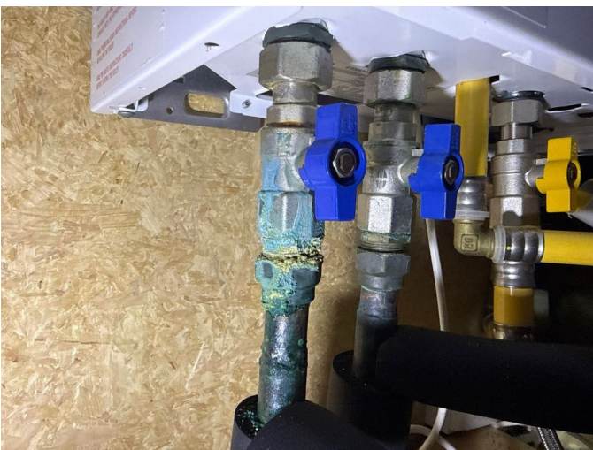
Another example of oxidation beneath the boiler
