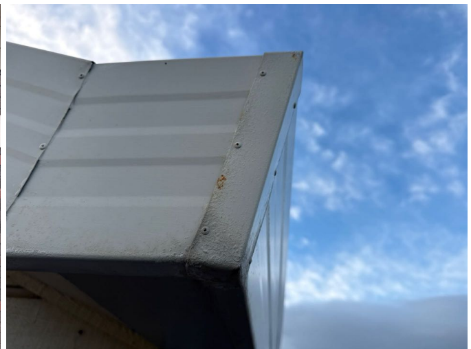
Example. There is surface rust to the steel fascia which requires attention
