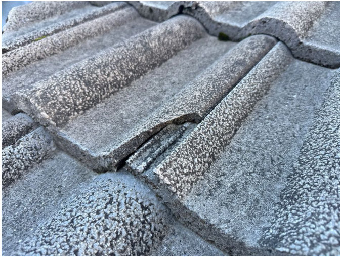
Example. Small sections of damage to the tiles like this are not a weather tightness risk.
