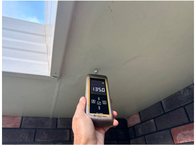
North side. Elevated moisture readings and bulge to the soffit. The owner disclosed a previous overflow which was caused by the failure of an expansion joint. There may still be moisture present in the soffit. A hole should be drilled to allow any pooling water to escape (if present).
