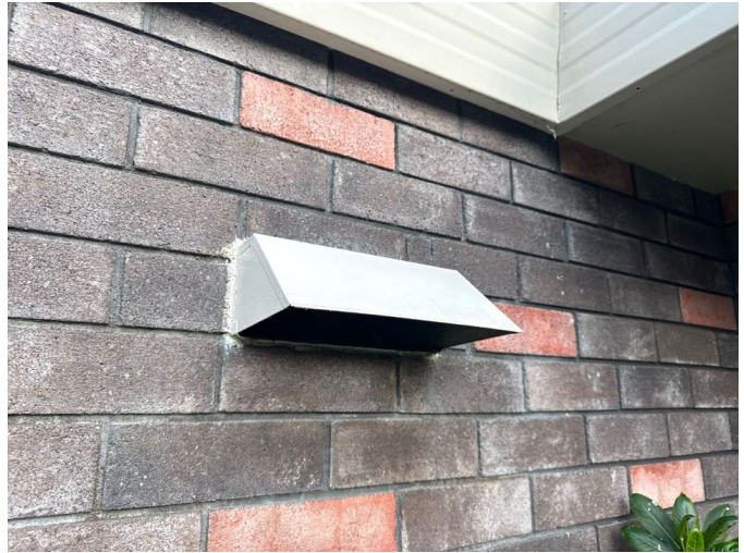
Extraction vents exit through the wall and soffits
