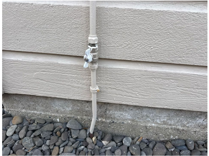
Water isolation valve to the southwest side
