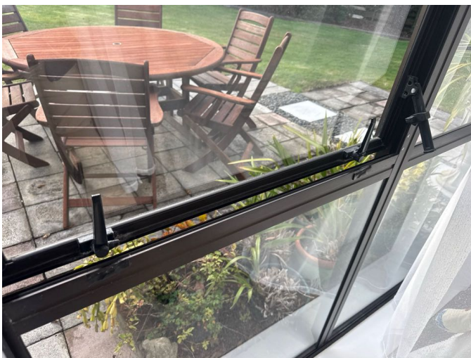
The windows are functioning in a typical condition for the age
