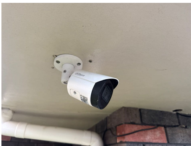
Security camera system installed. Untested.
