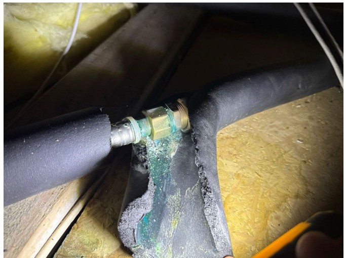
Oxidation to the pipe connections beneath the boiler and moisture staining. The owner advised that the system is to be serviced soon therefore the condition should be checked by the gas fitter/plumber then.
