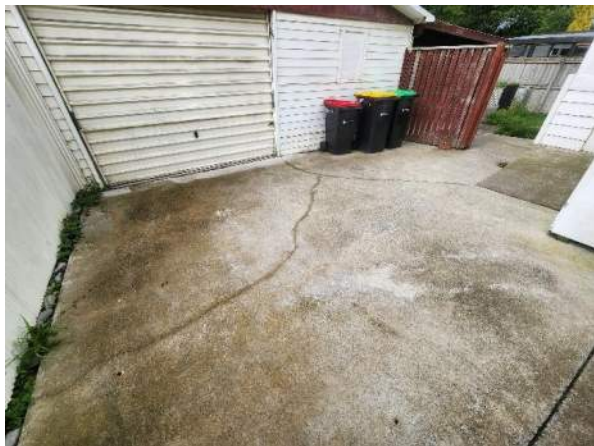
Figure 4: View of minor cracking to the concrete driveway adjacent to the garage looking southwest
