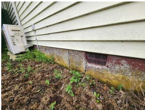
Figure 10: View of cracking to the perimeter beam on the west elevation
