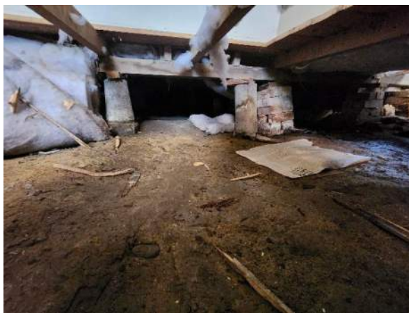
Figure 8: View of the mismatched piles in the subfloor
