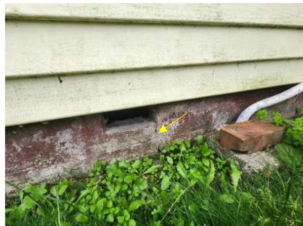
Figure 11: View of cracking to the perimeter beam on the south elevation
