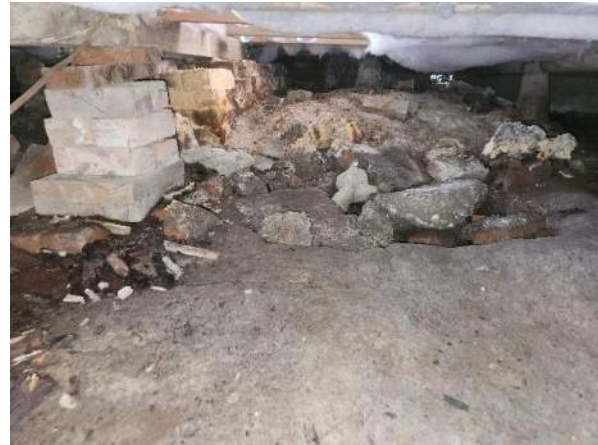
Figure 7: View of fill material (inferred construction waste) in the subfloor
