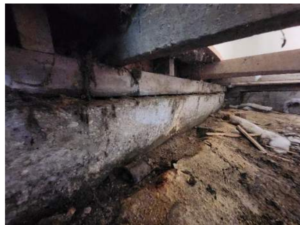
Figure 9: View of the overturned perimeter foundation in the subfloor
