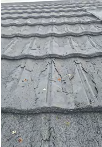
An example. Isolated patches of the roof cladding is missing the stonechip coating.
