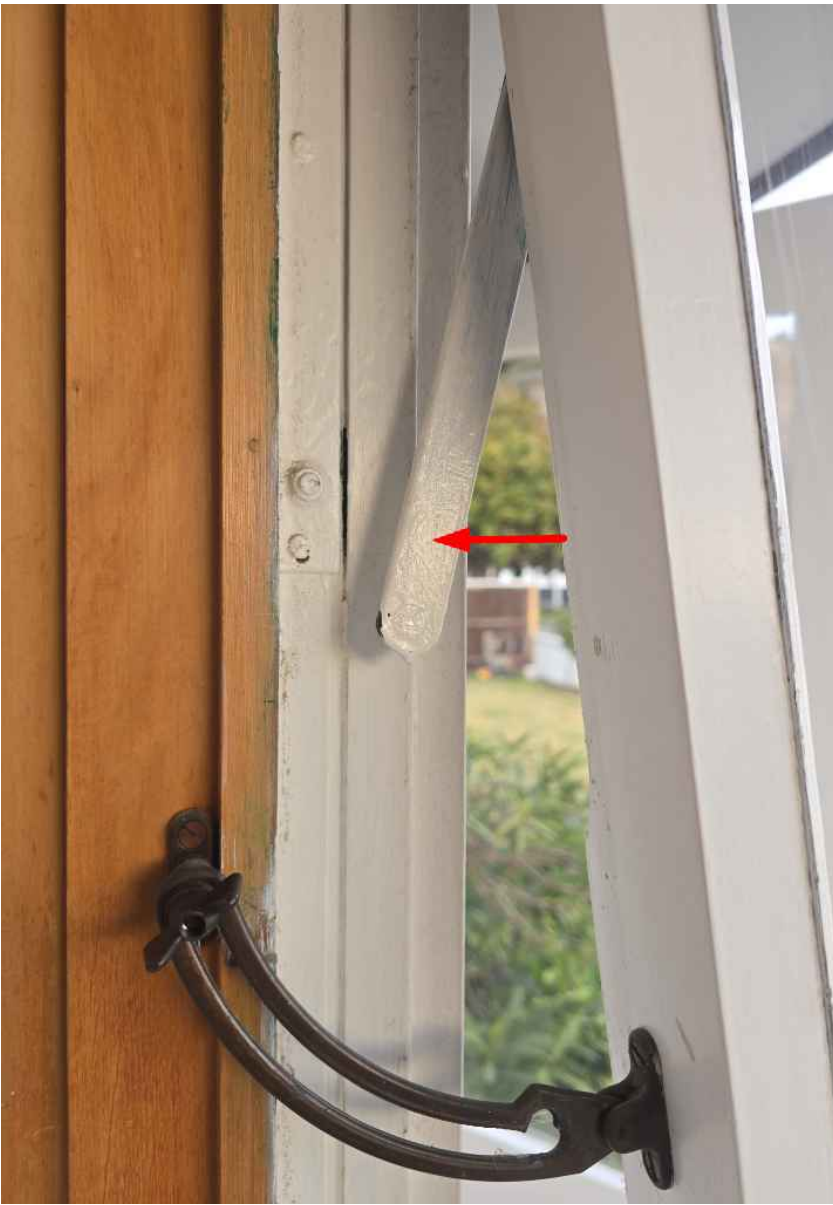
The living room window latch is broken.
