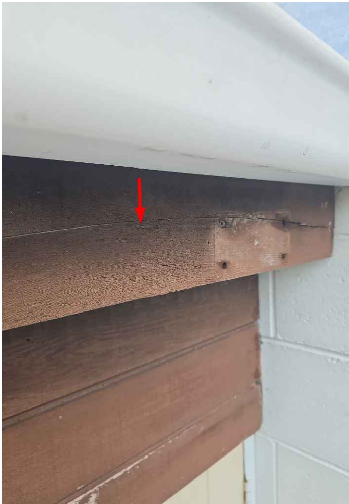
The fascia above the back external garage door has split.
