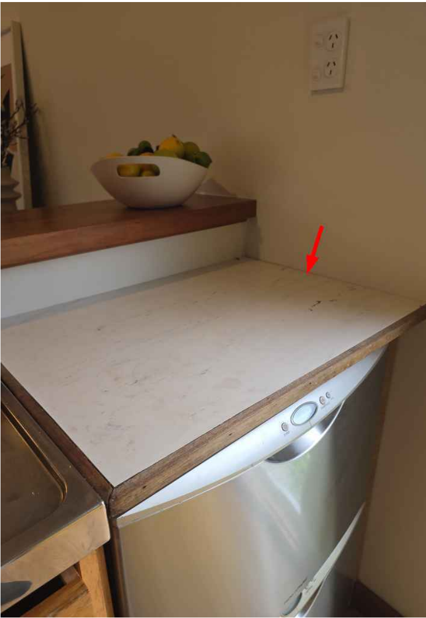
The kitchen bench top is loose.
