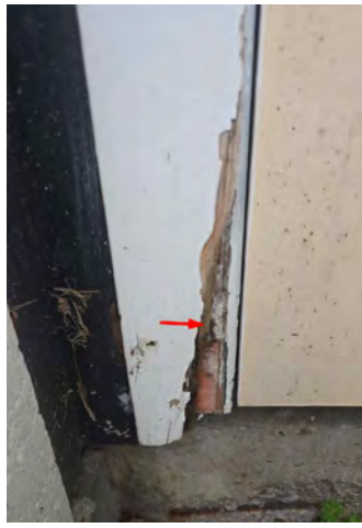
Rotten timber on the external garage door trim.
