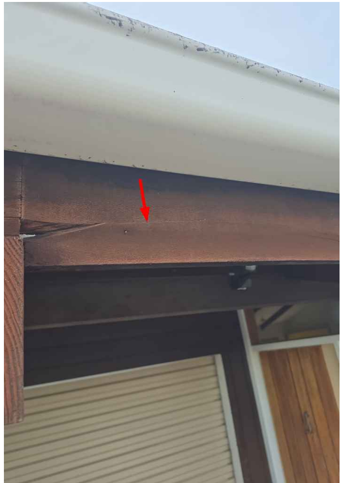
The fascia board above the garage has split.
