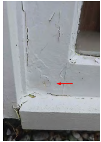
Evidence of repairs to the south side window frame.
