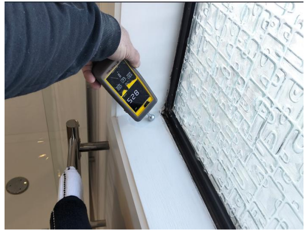
Elevated and wet moisture readings
