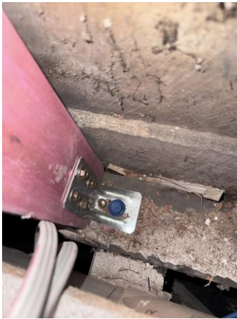
Photograph 17 – Angle-bracket connection to bearer (subfloor)
