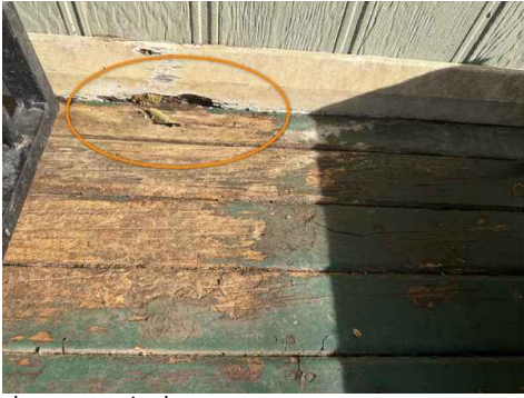
decay to timber
