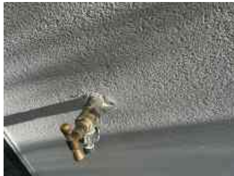
Recommend additional PVC flanges.
