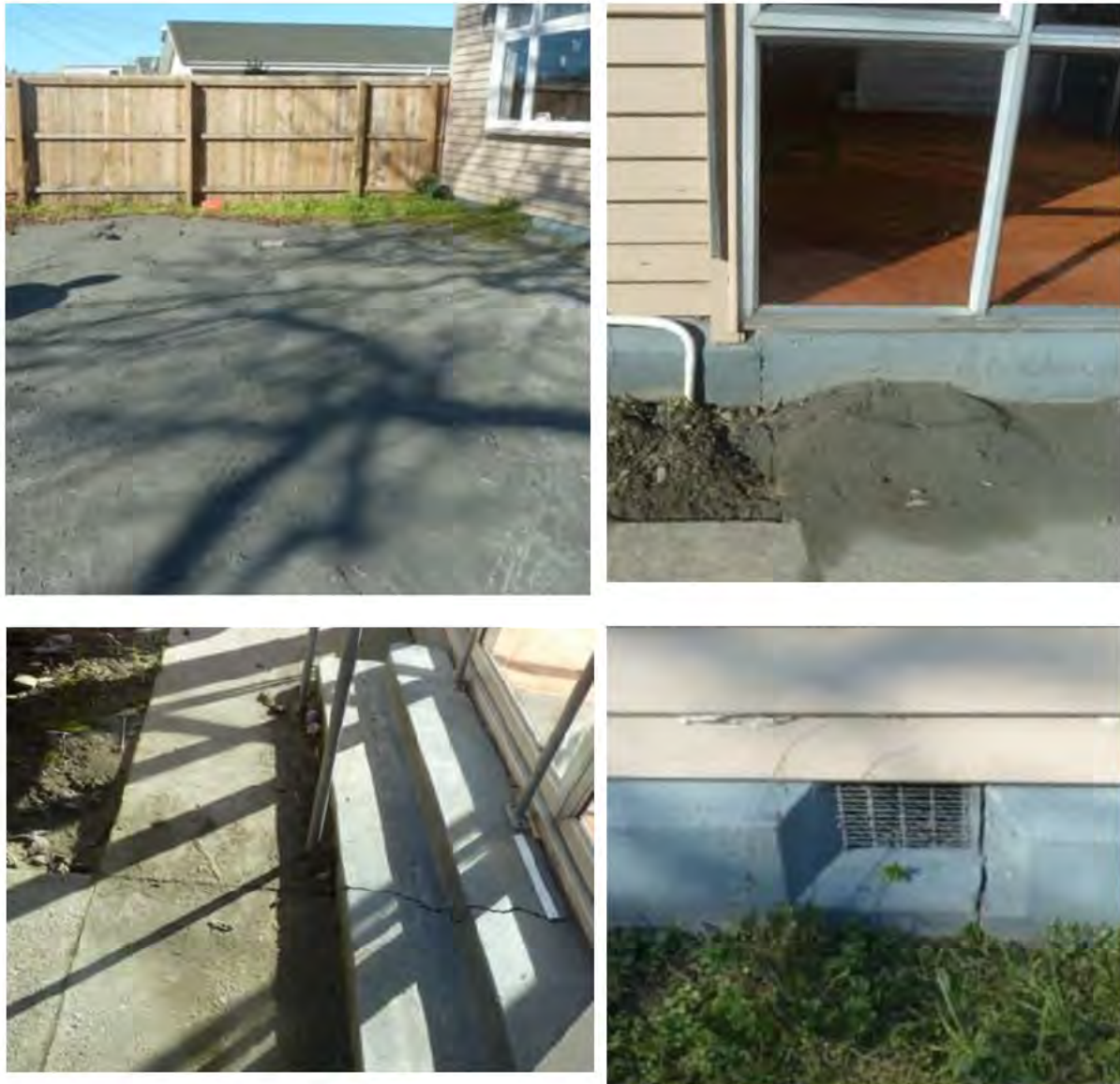
Figure 3 Sample photographs from EQC land team showing liquefaction ejecta around property and foundation damage
