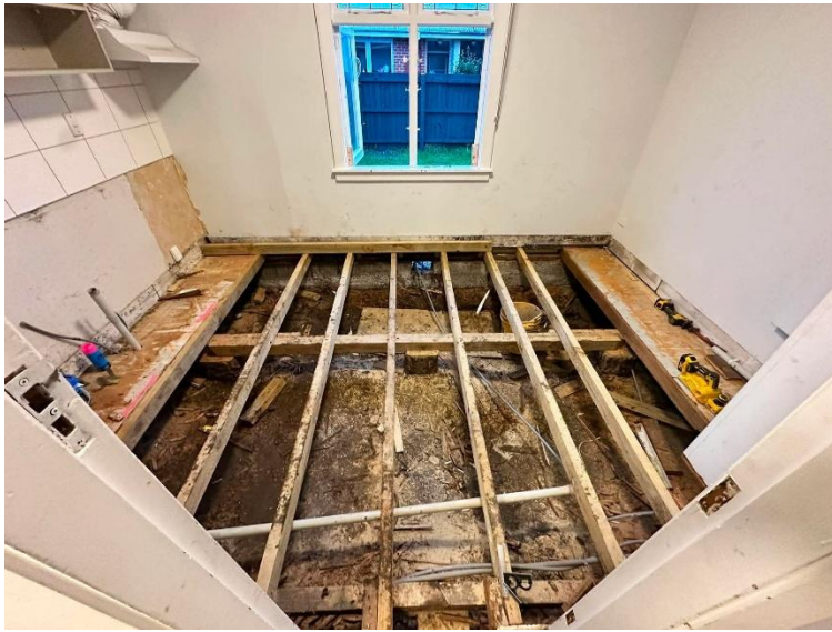
Ground level too close to floor – damaged joists replaced floor level adjusted to level
