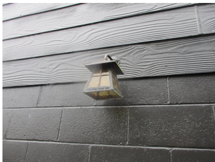
exterior lighting noted
