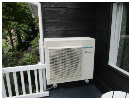
exterior air conditioning unit
