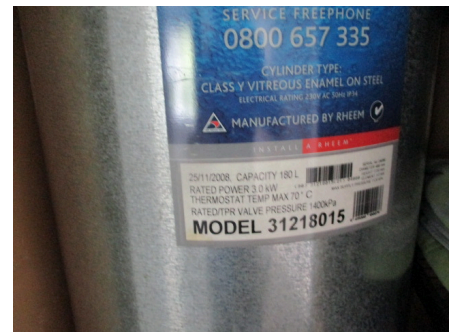
hot water cylinder
