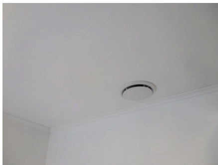
ventilation system downstairs
