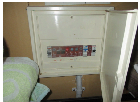
circuit breaker board
