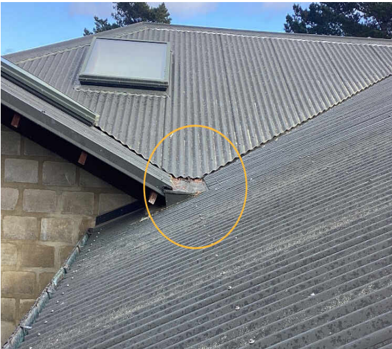
Approximate location above where stains were noted.
