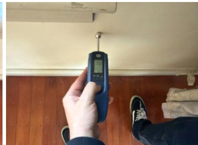
Dry reading around joinery
