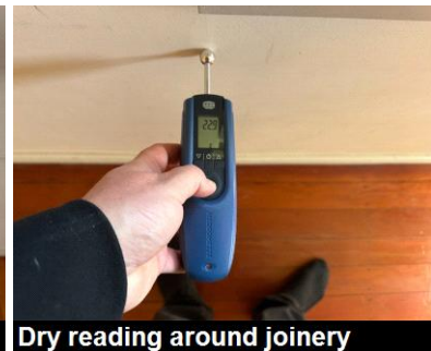
Dry reading around joinery
