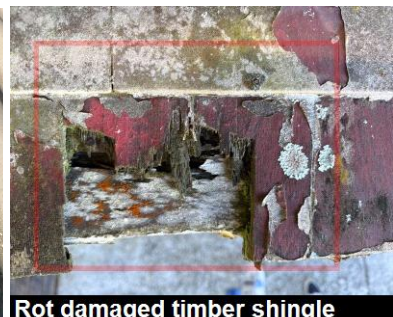
Rot damaged timber shingle roof
