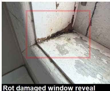
Rot damaged window reveal
