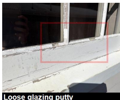
Loose glazing putty
