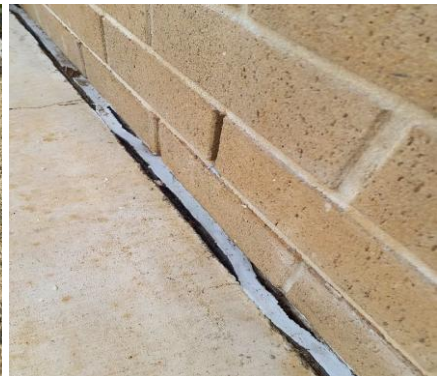
Driveway has separated from the wall of the dwelling
