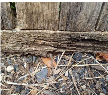
Wood decay to retaining wall timbers
