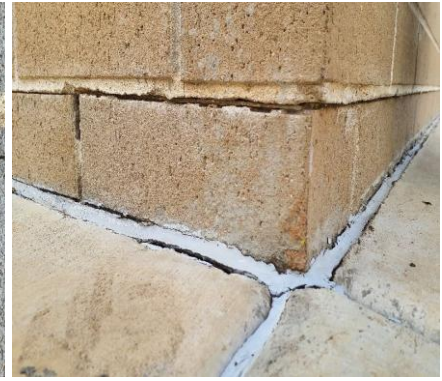
Cracking to mortar at damp course level
