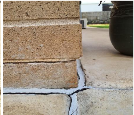
Signs of movement to the brickwork
