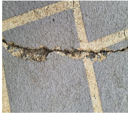
Cracking to the path
