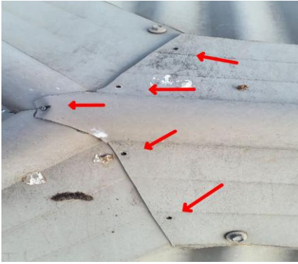
Pop rivets missing from joins of ridge capping
