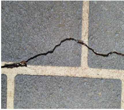
Cracking to the driveway
