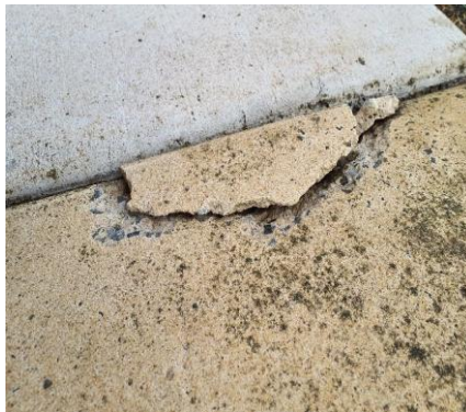
Section of path has broken away
