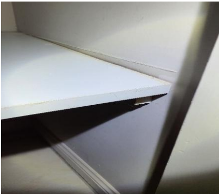
Support for linen cupboard shelf has separated
