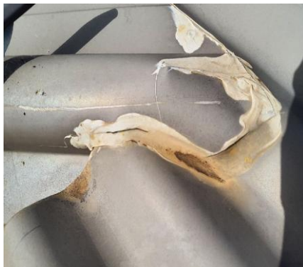
Sealant has split on join of ridge capping
