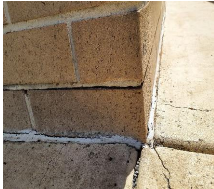
Signs of movement to the brickwork
