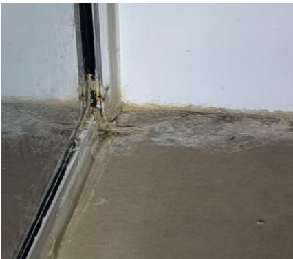
Leakage from the bathroom shower recess
