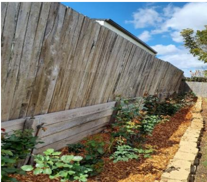
Retaining wall and fence is leaning
