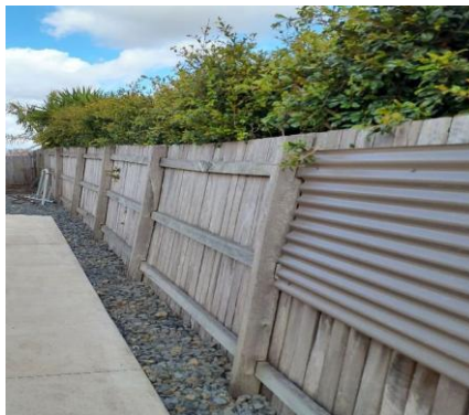
Fence and retaining wall are leaning
