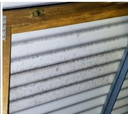
Mould to underside section of the roofing iron
