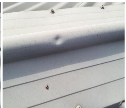
Hail indentations to the roof exterior
