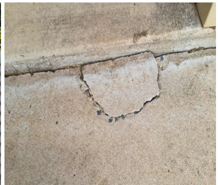
Section of the driveway has broken away
