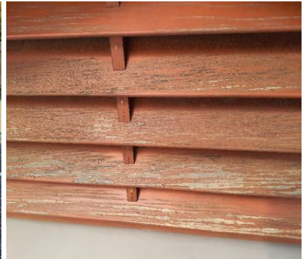
Weathering to timber work in the gable
