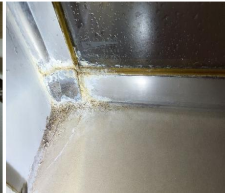
Sign of leakage from the ensuite shower frame
