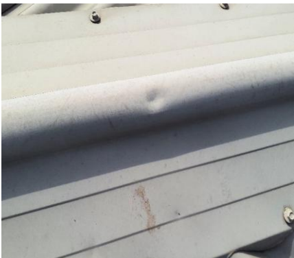
Hail indentations to the roof exterior
