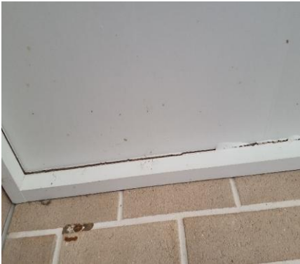
Timber moulding has separated slightly from the patio ceiling
