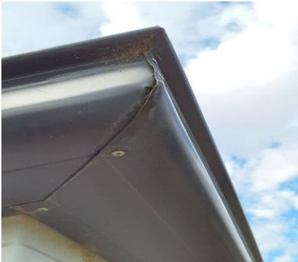
Gutter is leaking on join
