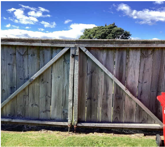
We recommend front gates leading into property are adjusted for ease of operation
