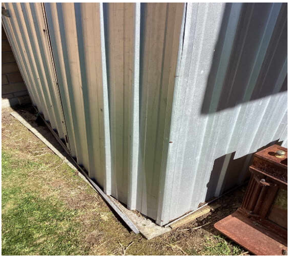
The shed appears to be twisted out of shape.
