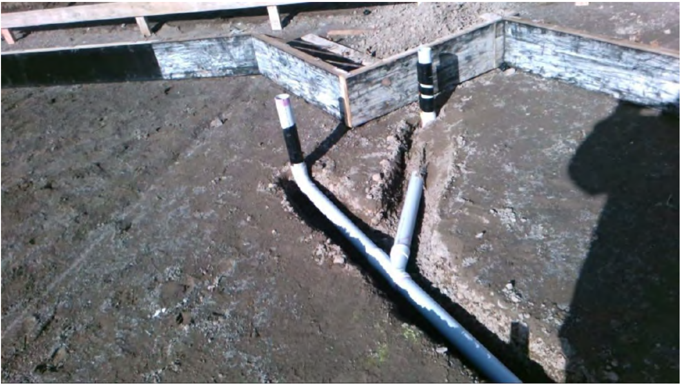
waste pipes filled with water and wrapped Taken at 3:04 PM on Wednesday 22/08/2018
