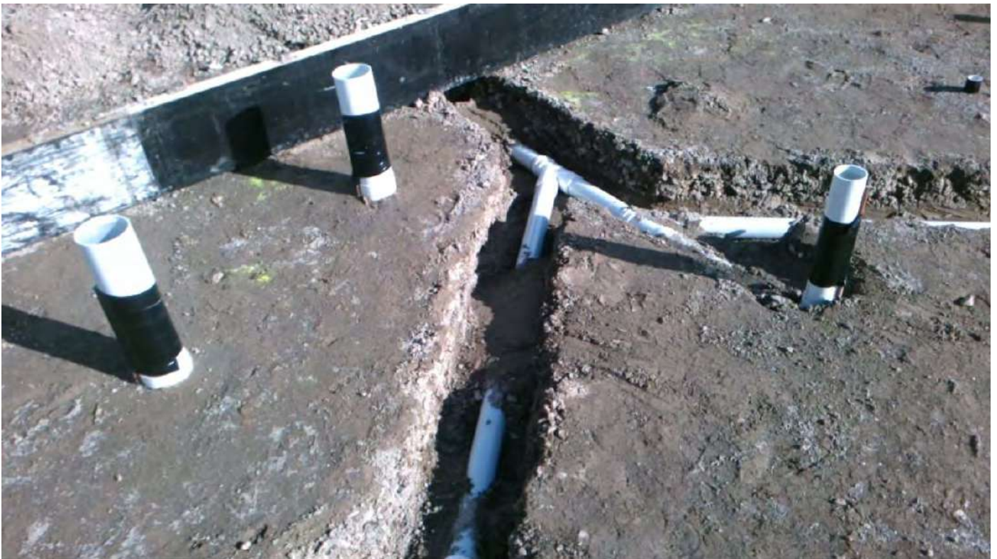
wc and grey water waste pipes Taken at 3:04 PM on Wednesday 22/08/2018
