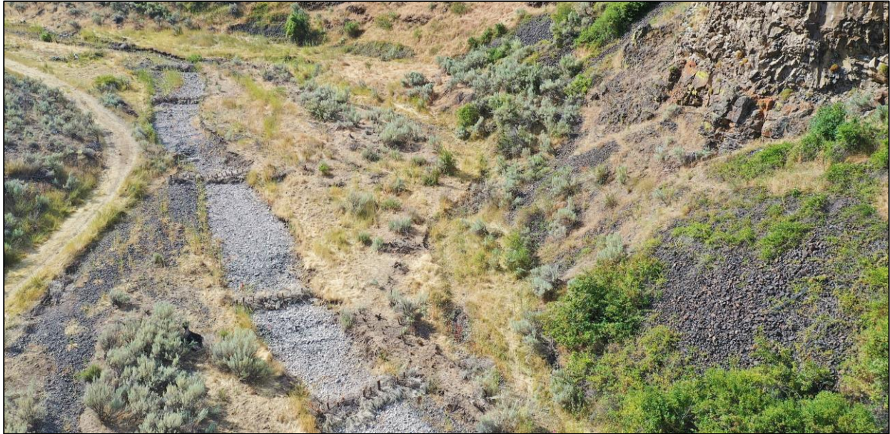
FIGURE 8. A SERIES OF BDAs CONSTRUCTED FROM LOCALLY HARVESTED SAGEBRUSH AT THE UPPER EXTENT OF THE WILSON / SMITH LT-PBR PROJECT. MUCH OF STRUCTURE CONSTRUCTION WAS DONE DURING DROUGHT PERIODS WHERE SURFACE FLOW WAS ABSENT.
