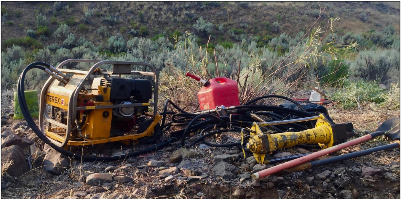
FIGURE 26. TYPICAL HYDRAULIC POWER SOURCE AND POST POUNDER USED TO DRIVE POSTS REQUIRED FOR CONSTRUCTION OF BDAs.
