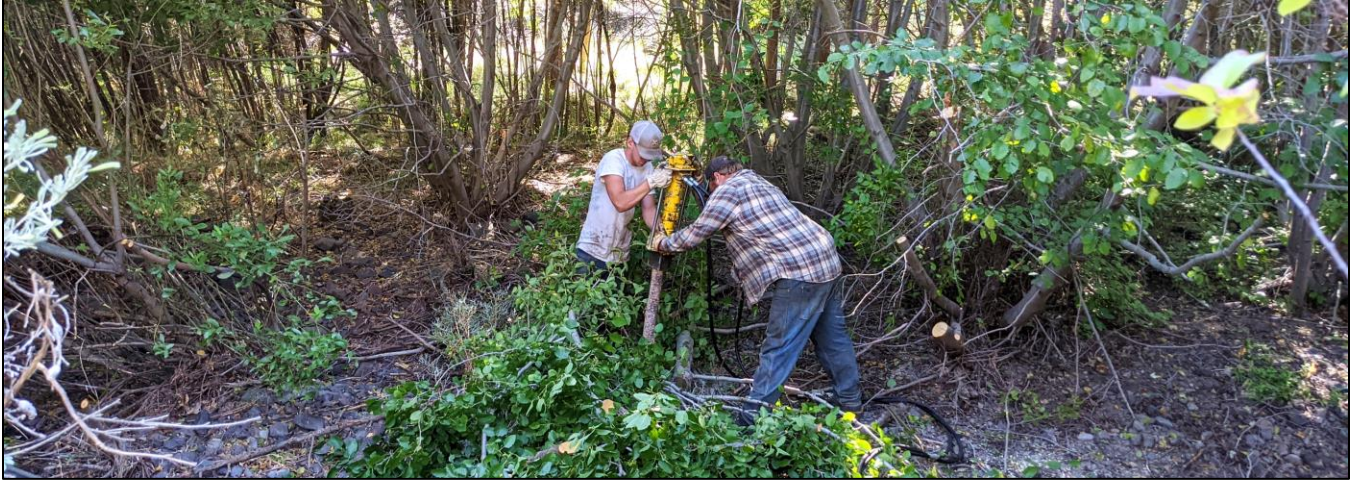
FIGURE 7. JT HAND AND KYLE HAND INSTALL SUPPORTING POSTS TO A NEWLY INSTALLED PALS IN THE LOWER SMITH REACH OF THE THIRTYMILE – WILSON / SMITH LT-PBR PROJECT.
