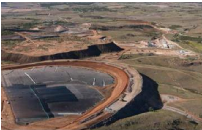
Figure 11 Construction of the tailings dam for Kanmantoo's mine located 25 km away from Mount Baker in the Adelaide Hills, Australia.
