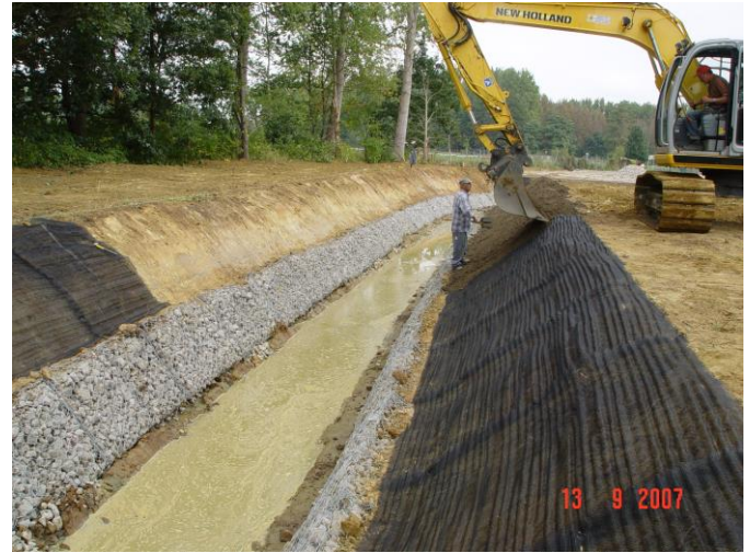
Figure 13 Laying of the topsoil on top of the geocomposites in one of the canals
