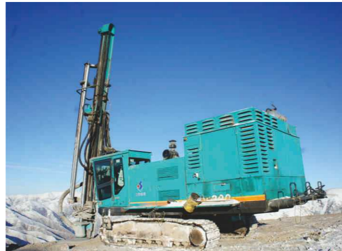
伊朗最大的铜矿施工(海拔2800米, 零下15°C) Construction in Iran's largest copper mine (the altitude of 2800 meters, the temperature of 15 degrees below zero celsius.)
