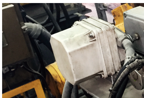
Antes: CAM switch mecánico. Before: Mechanical cam limit switch.
