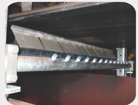
Razor-Back MDX with spray bar attachment is installed for more efficient cleaning at this iron ore facility.
