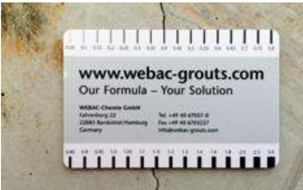
Measuring the crack width
