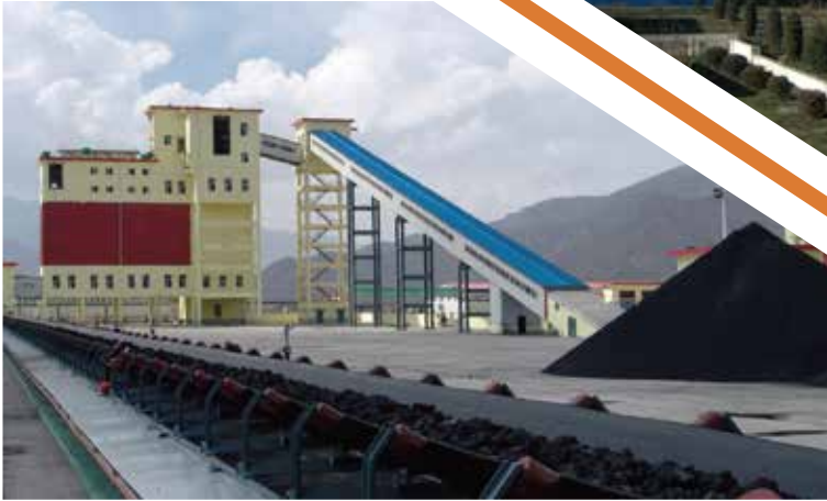
Shanxi Shuiyu Coal Handling Plant Belt Conveyor for Coal Handling Plant
