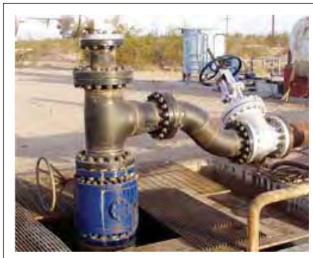
Master Valve Geothermal Brine
