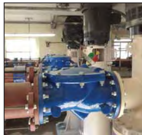
Crystal Springs Pump Station Roanoke, VA
