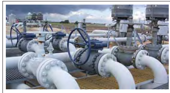
Salt Dome Brine & Gas Pumping Station
