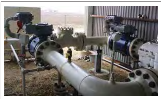
Crude Oil Pumping Station Pig Launcher/Receiver
