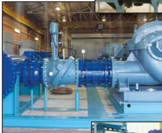
Tilted Disc® Check Valve on Discharge of Centrifugal Pump.
