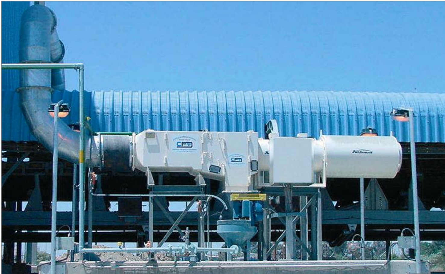
Wet Scrubber at a diamond mine in Jwaneng, Africa
