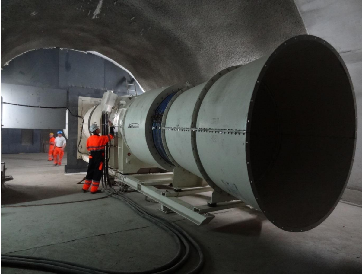
Main fan in the Gotthard base tunnel, Switzerland Impeller diameter: 1.80 m; power: 630 kW; speciality: 100 % reversible
