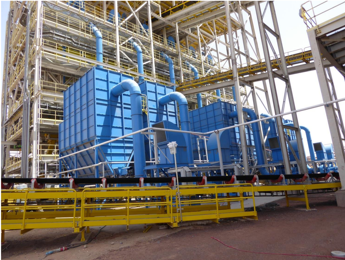
Bag filter systems in a surface mine in Mauretania Air flowrate: 22 filter units with a total volume of 631,600 m 3 /h
