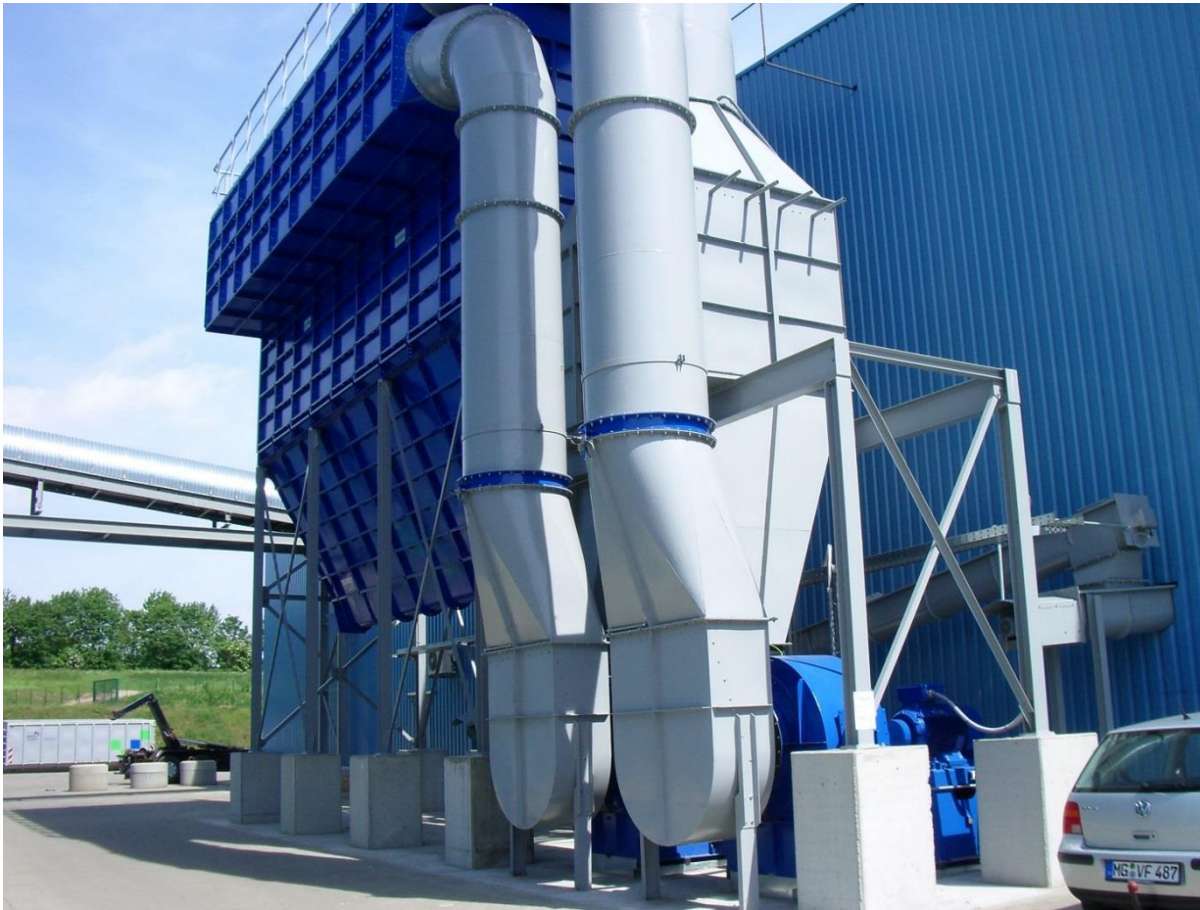
Bag filter system in a waste sorting plant in Neuss, Germany Air flowrate: 130.000 m 3 /h
