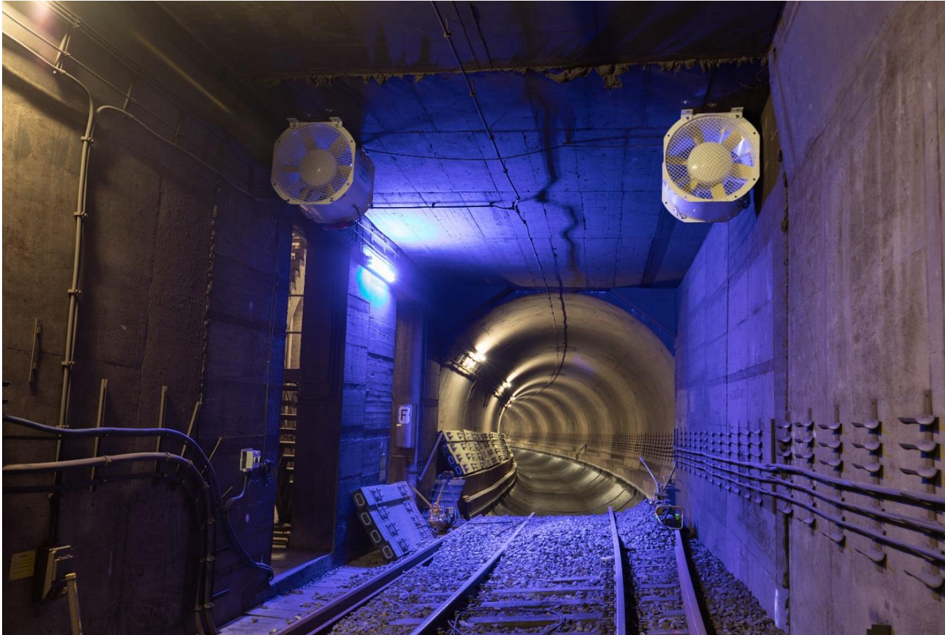
Dedusting and ventilation in a metro tunnel in Munich, Germany
