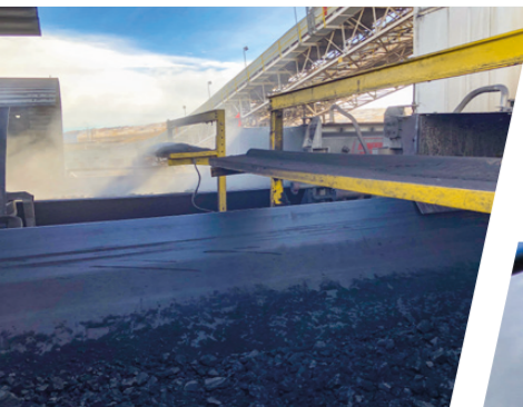
STEINERT Metal Detector in a coal wash plant
