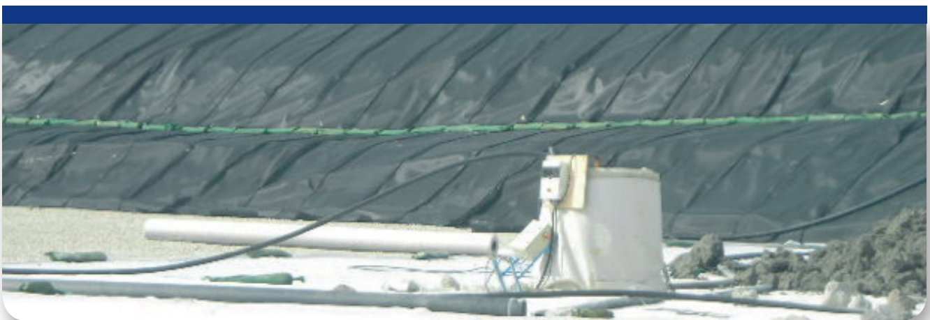
Fig. 8. Detail of AM5 composite installed on slopes. No normalizing layer is generally needed on slopes.
