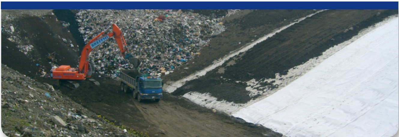
Fig. 5. General overview of Balleally landfill under operation. The waste is disposed when the new cell is still being constructed. Normalizing layer is clearly seen above the drainage composite for leachate collection.
