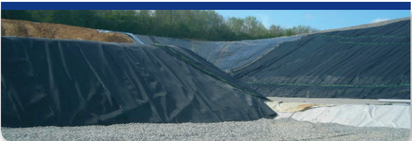
Fig. 7. In Tourville landfill, gravels were used as a normalizing layer over the drainage composite. The use of a drainage composite reduced 3 times the need of gravels.
