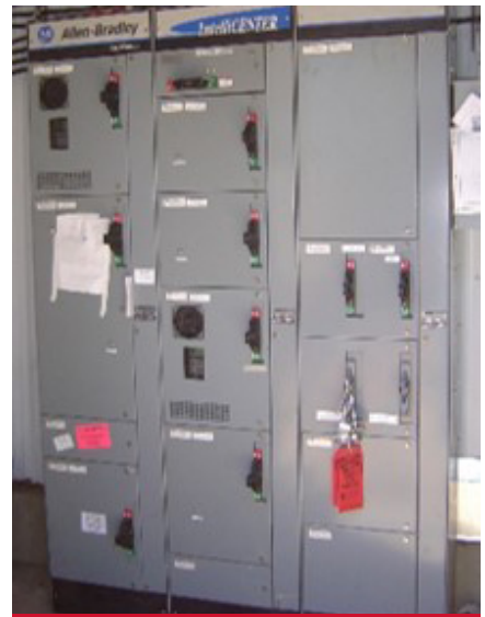
Motor Control Center
