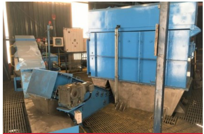
Two Stage Falling Stream-Based Sampling System
