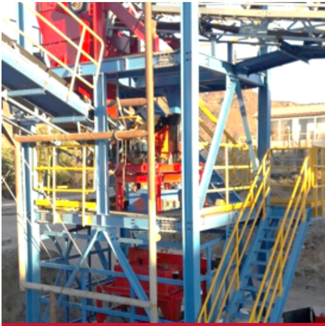
Falling Stream Sampler-Based Two Stage Sampling System
