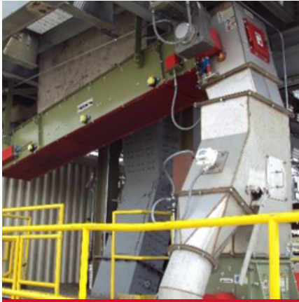
Automatic Diverter Gate for Crusher Bypass
