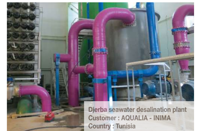
Djerba seawater desalination plant Customer : AQUALIA - INIMA Country : Tunisia
