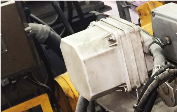
Antes: CAM switch mecánico / Before: Mechanical cam limit switch
