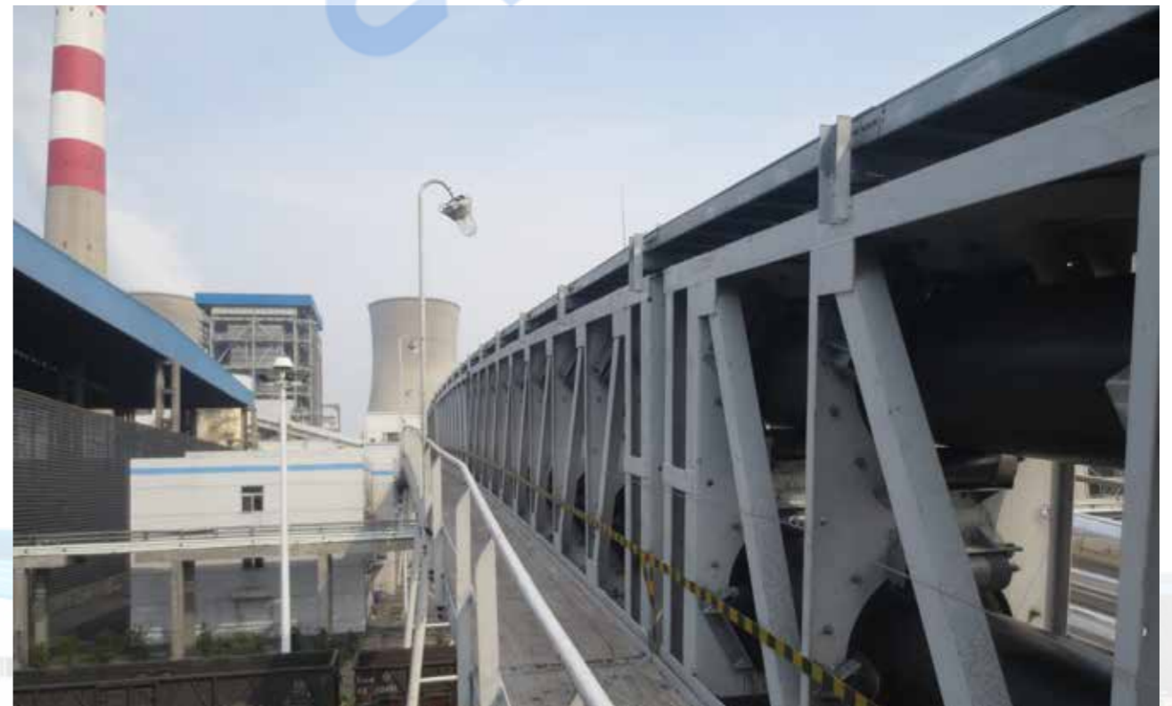
Kaifeng Power Plant , China
