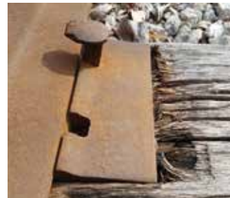
Lifted spikes between the rails
