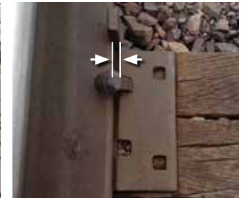
Rail base and tie plate gap
