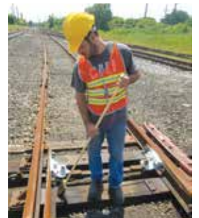
Track Switch Maintenance
