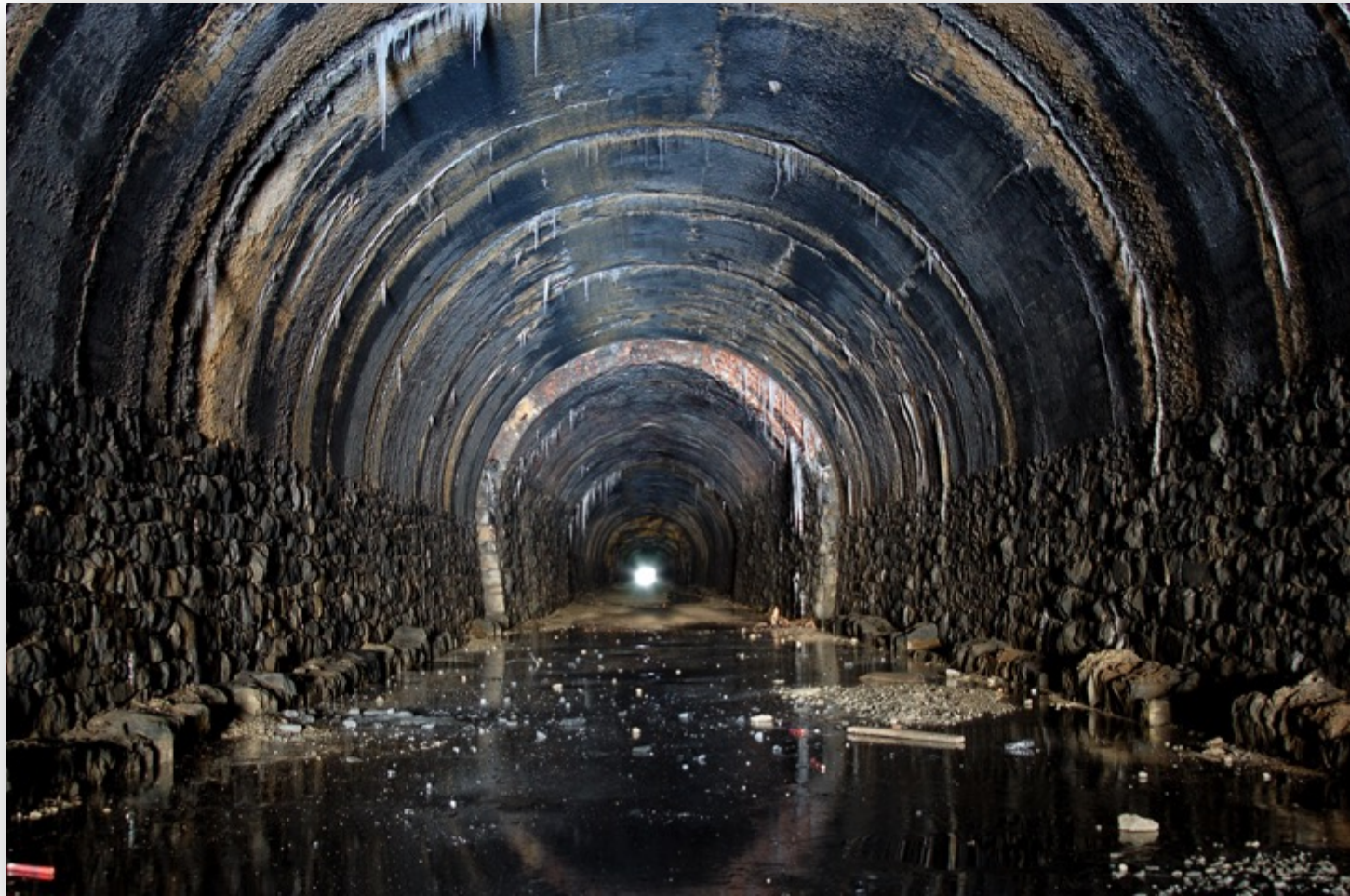
Original Pattenburg Tunnel: Once used as a Mushroom Farm, Now it is used by RR MOW Trucks
