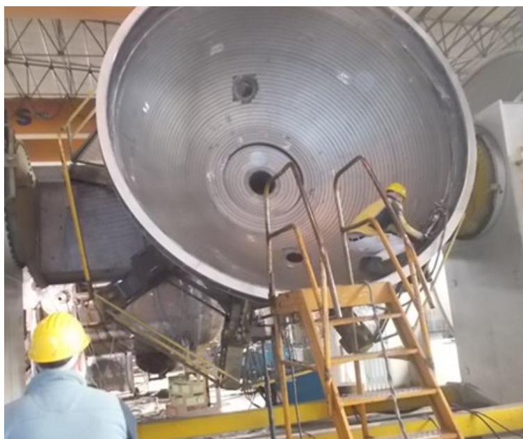
At left, a worker inspects the bottom head of a reactor vessel as it’s being manufactured. The vessel will be installed at the refinery next year.
