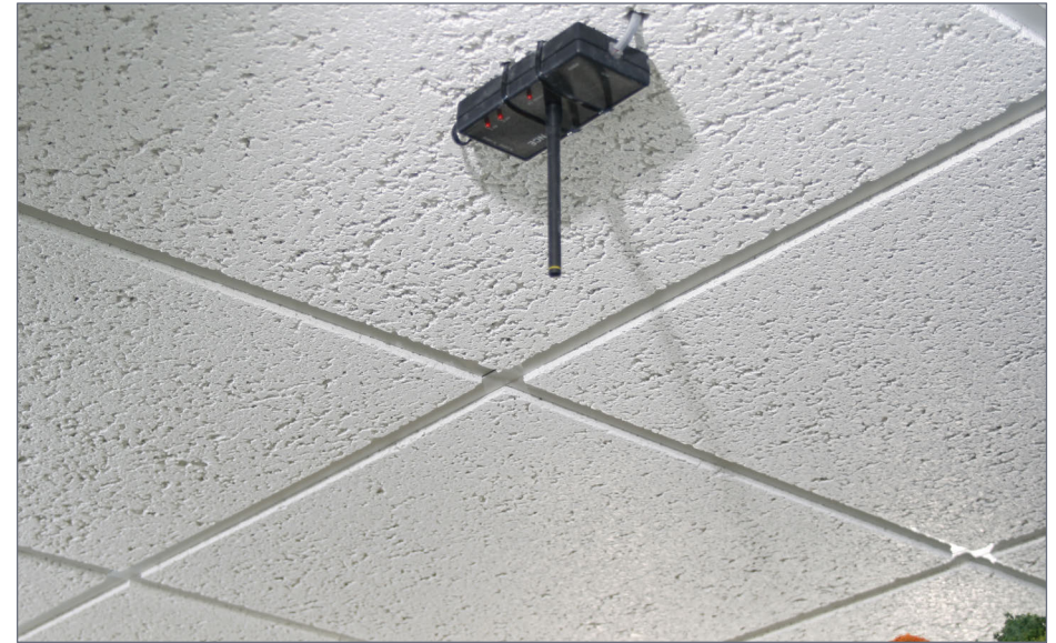
25. I mounted the NCE RB02 radio antenna on the ceiling for better coverage. I also installed a radio repeater to cover my zig-zag basement space.
