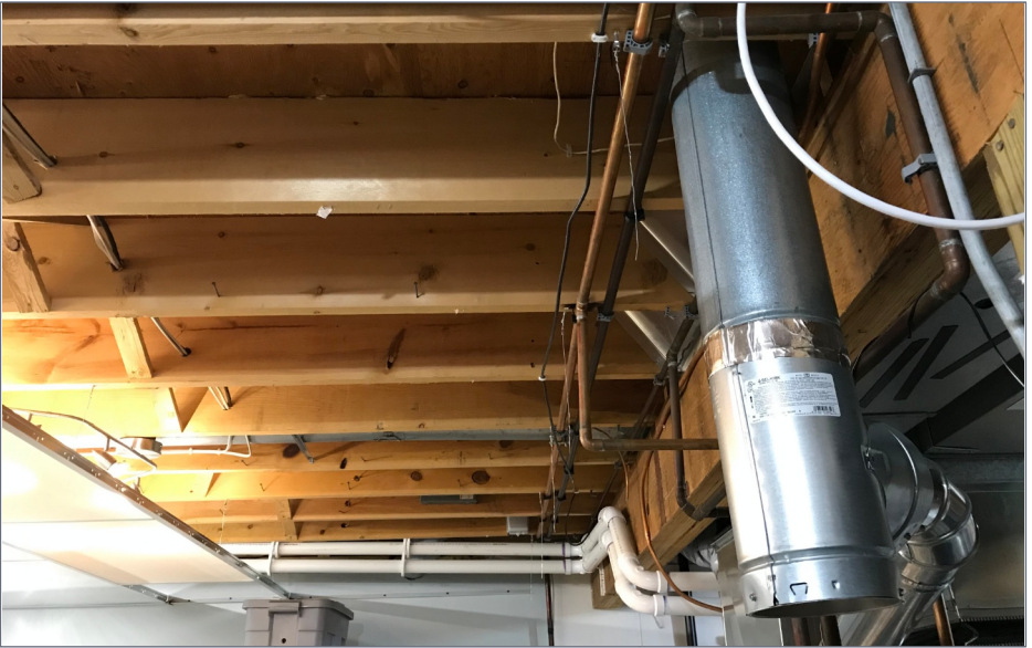
2. Exposed floor joists and utilities create a visual mess that detracts from the layout.
