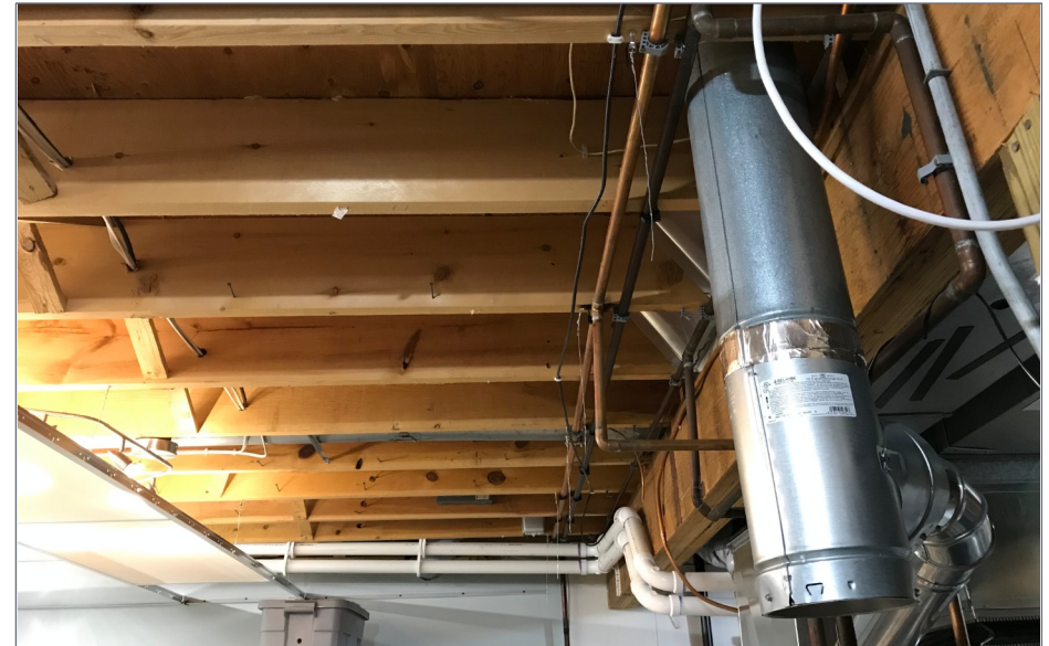
2. Exposed floor joists and utilities create a visual mess that detracts from the layout.
