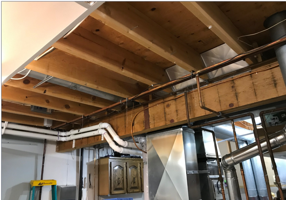
7. Working around pipes made designing a framed wall nearly impossible without severely cutting into the already limited layout space.
