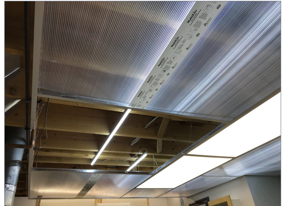
11. LED light panels are more versatile than fluorescent. Some brands have built-in switches to adjust color temperature, and most are dimmable.
