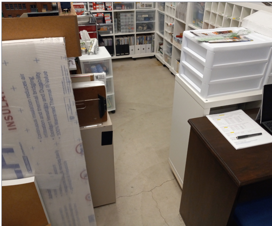
4. Bare concrete floor is difficult to keep clean. Cracks and stains make it unattractive.
