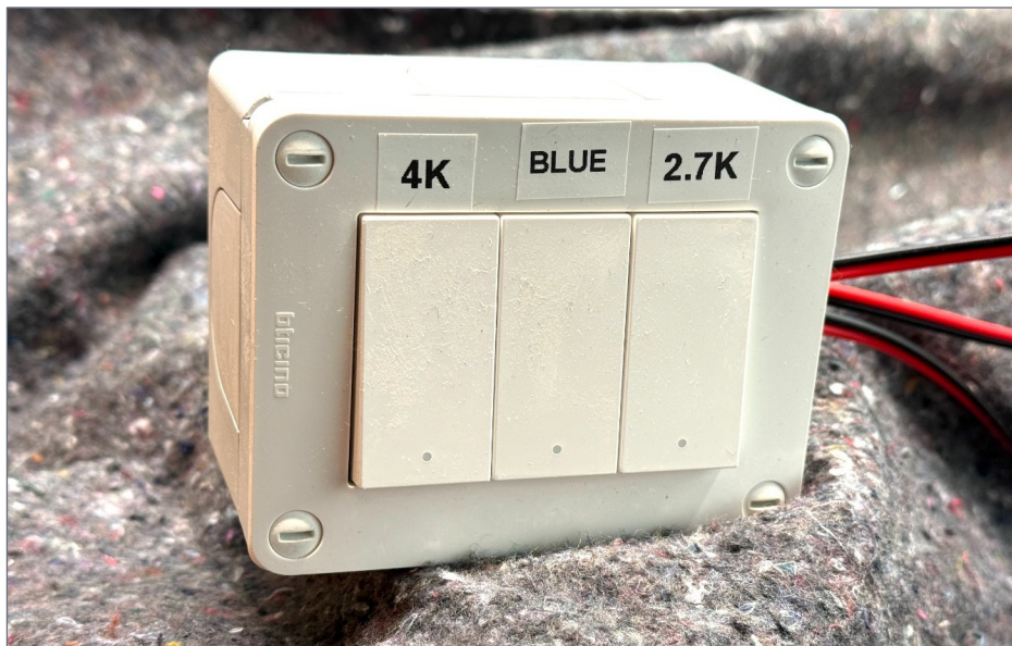
11. Here is the control switch box for the three LED light strips. I can turn on or off any combination.
