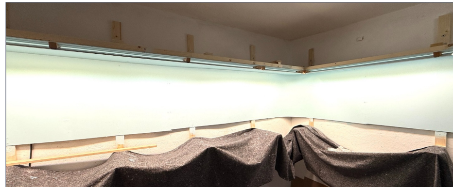
12. When the 2700K and 4000K strips are both on, I get bright medium-white lighting shown here.
