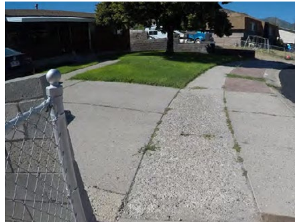
Spalling on sidewalk in Magna
