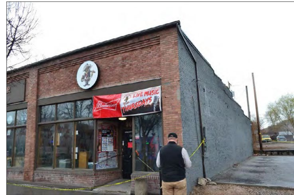
30 of 56 9071 and 9075 West Magna Main Street, contributing, after earthquake, north and west elevations, facing south-southeast. Photographer: S. Cornell Date photographed: 3/24/20
