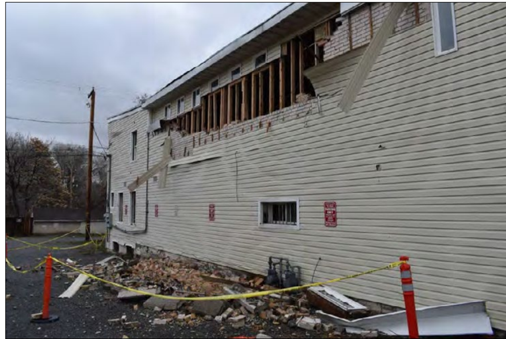
37 of 56 West elevation of 9108 West Magna Main Street, contributing, after earthquake, west elevation, facing north-northeast. Photographer: S. Cornell Date photographed: 3/24/20
