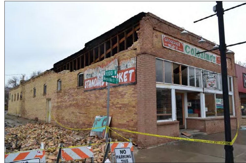
14 of 56 9009 West Magna Main Street, contributing, with earthquake damage, north and east elevations, facing southwest.
