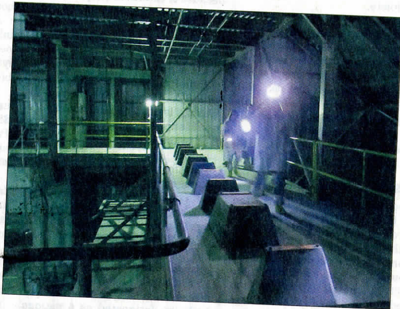
Courtesy Oregon Department of Energy Hanford officials and invited visitors take a look above the H Reactor core when the reactor was recently unsealed for an inspection required every five years.
