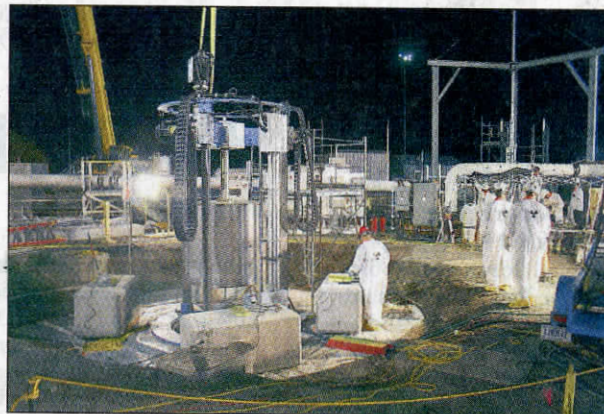
The dome of Hanford Tank C-105 was cut open in June 2013 to allow the Mobile Arm Retrieval System to be lowered through a larger riser into the tank.
