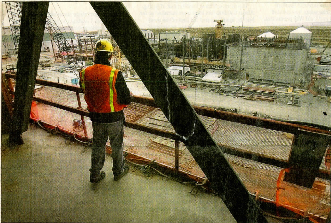
Greg Atencio of Bechtel National looks over progress at the Hanford vitrification plant. The massive project has reached the 50 percent completion mark for combined design and construction. See photo galleries at tricityherald.com .
