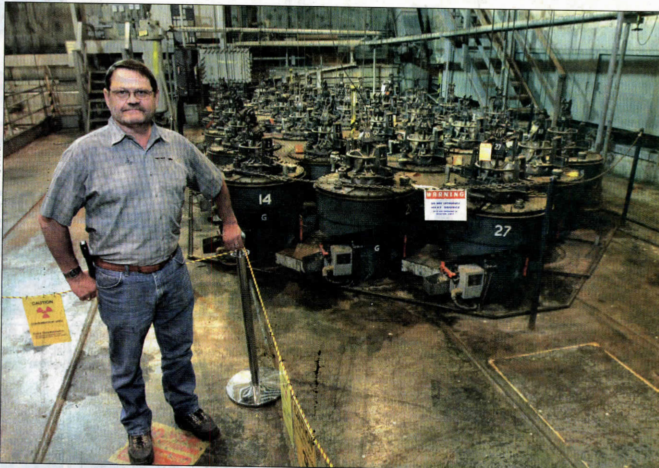
Russ Fabre, B Reactor tour manager, stands next to a cluster of 29 vertical boron-infused safety rods hung above the reactor. In the event of a malfunction, the rods would be lowered into the core and shut down the reactor's chain reaction. See three galleries of contemporary and historical Hanford photos at www.tricityherald.com .
