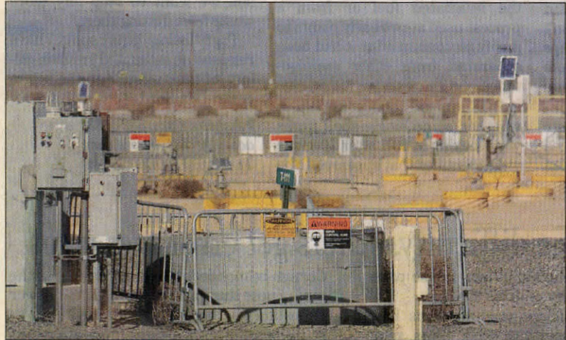
Hanford single-shell Tank T-111 is potentially leaking up to 300 gallons of radioactive waste per year.
