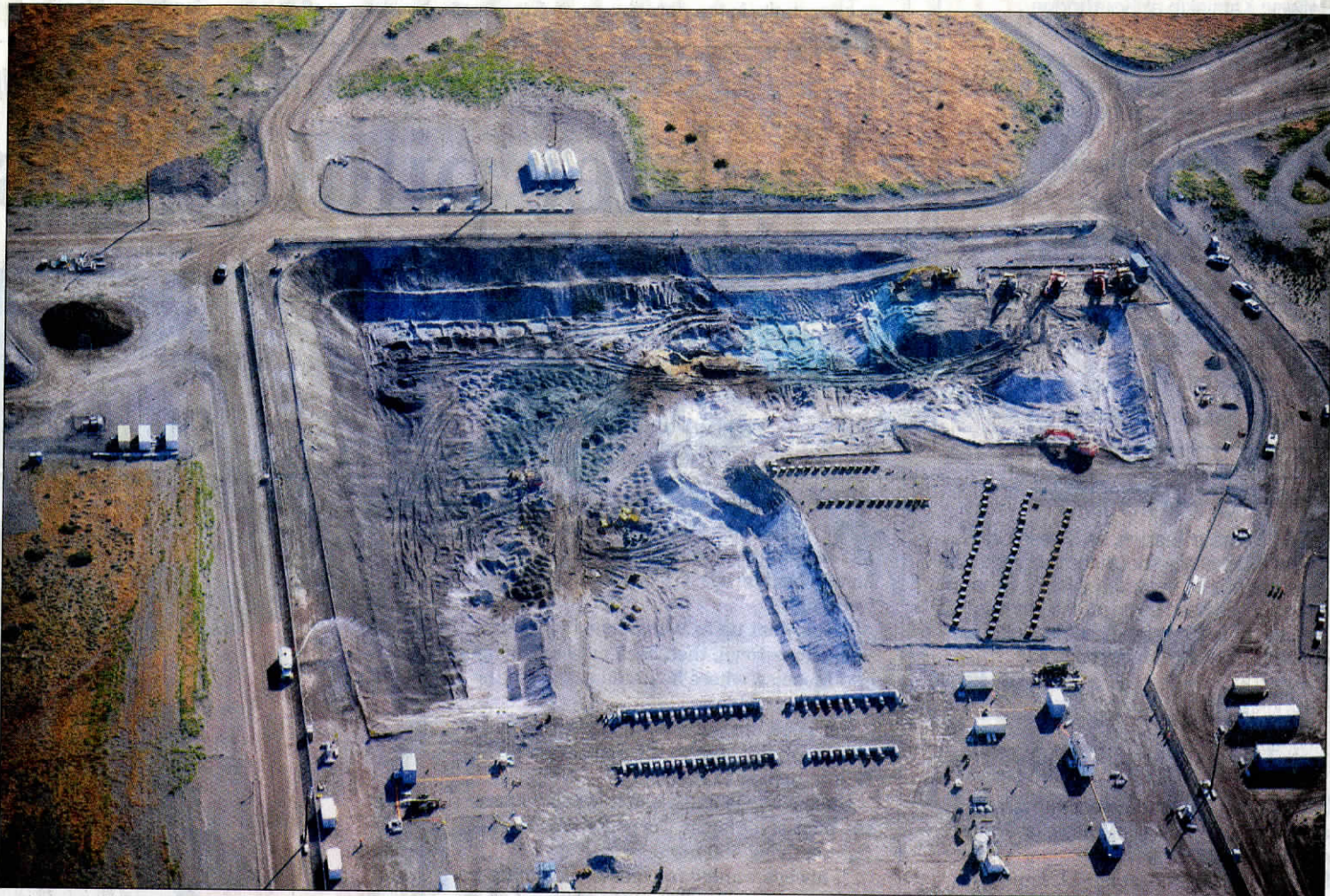
Work is close to being completed to dig up the high-hazard waste trenches at Hanford's 618-10 Burial Ground.
