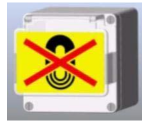
Scan room quench button located behind door
