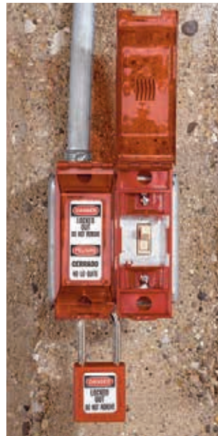
Wall Switch Lockout
