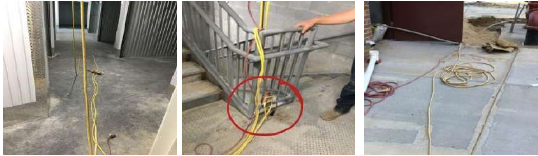
Several cords daisy chained in stairwell. Cords supplying power other than to workers on exterior of project.
