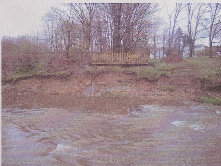
Bank Erosion Below Observation Deck
