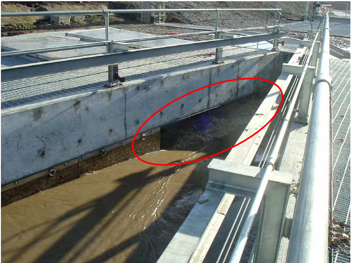
Figure 4.7. Picture Taken During January 2005 Flood Showing Fish Screens Removed in Robles Canal.
