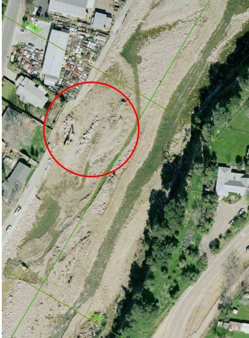
Figure 4.12. Aerial photo taken in February 2005 showing erosion of Live Oak Levee erosion between XC 9.375 and 9.4697.
