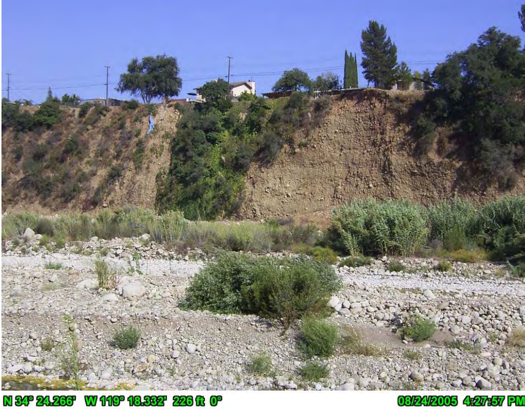
Figure 4.15. East Bank of Ventura River Located at RM 9.6 Showing Some Recent Bank Failure,
