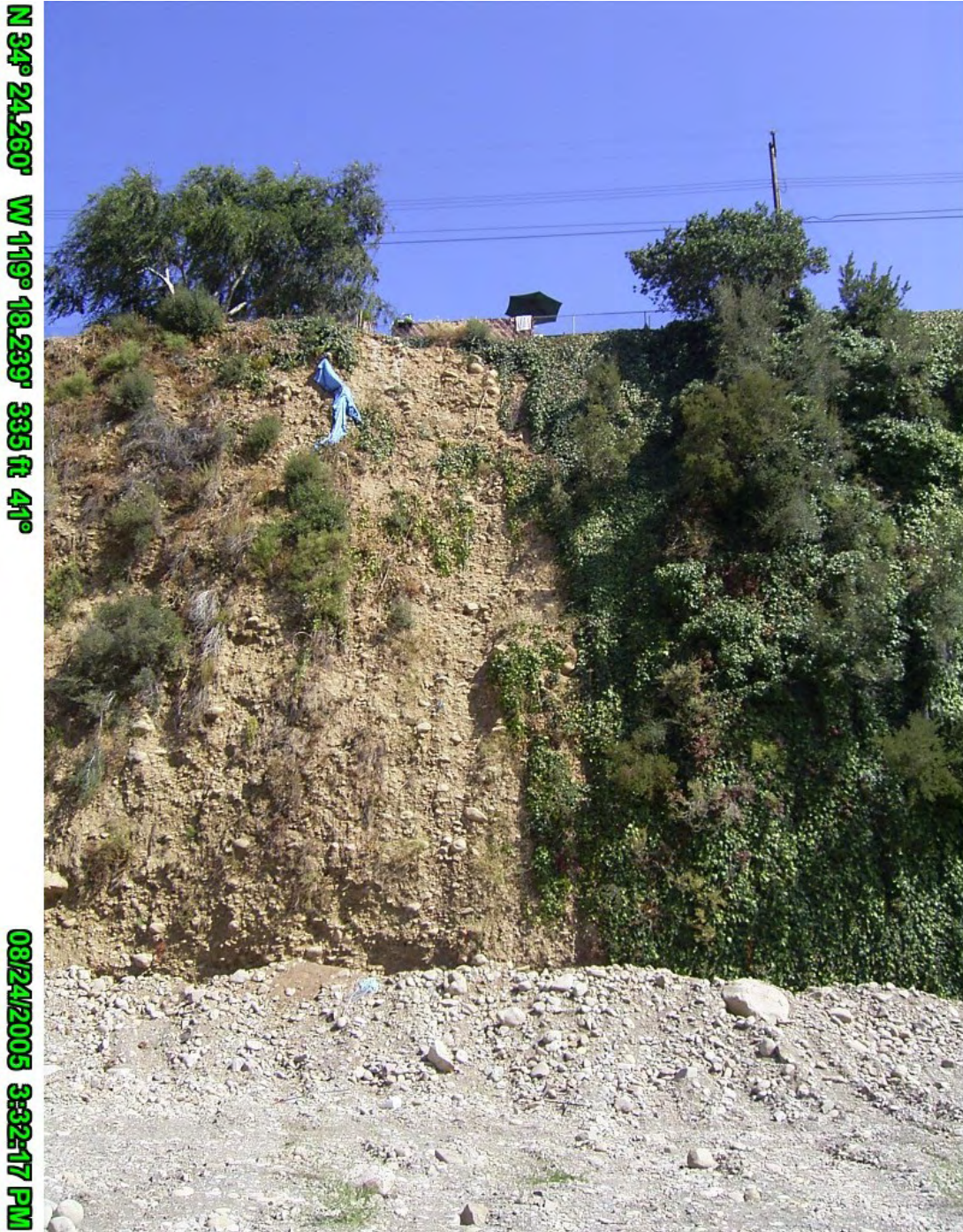
Figure 4.14. East Bank of Ventura River Located at RM 9.6 Showing Alluvial Material of Terrace and Some Recent Bank Failure.
